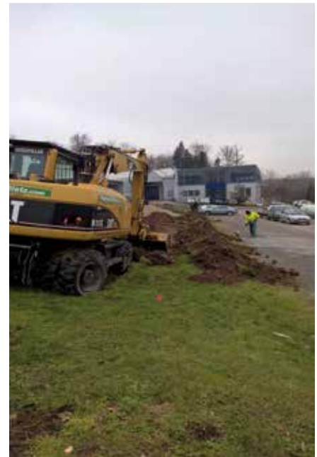
Start construction works, here the enlargement of the car park for the employees.
